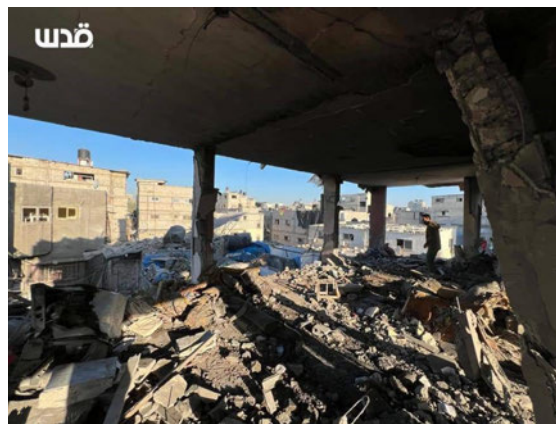
The remains of the Ghandour family home in Khan Younis after it was destroyed in an Israeli airstrike on December 3, 2023. © 2024 Quds Network
